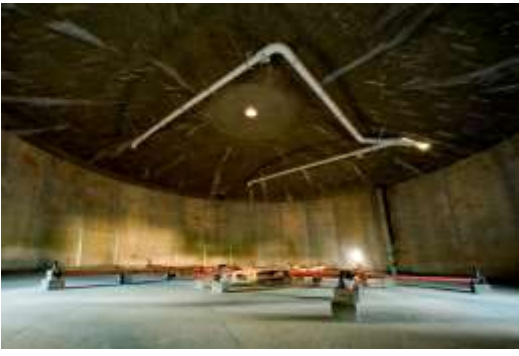
odor control and jet mix
