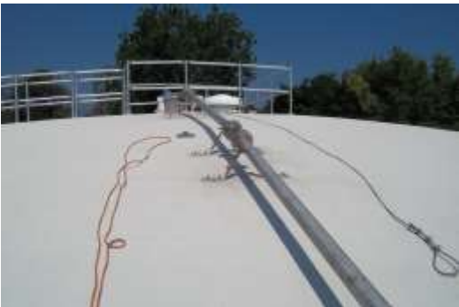
pipng on roof
