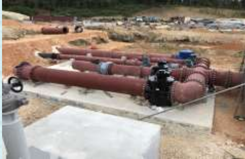
Influent Flow Distribution Piping
