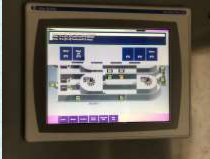
Ovivo Oxidation Ditch
